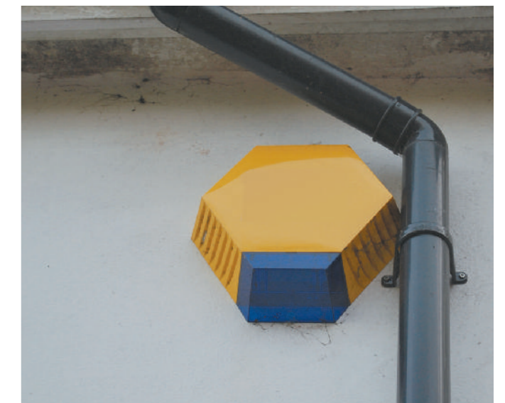
An alarm box is a powerful deterrent to burglary however professional burglars can tell the difference between a genuine and a dummy alarm system.
